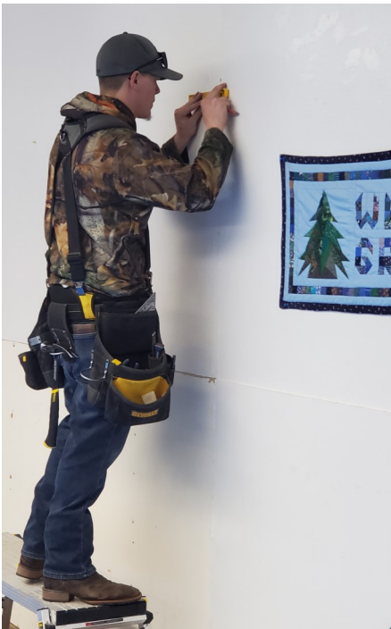
Joe Milner of Cottrell's Construction marks the spot for a new window in the Grange hall.
