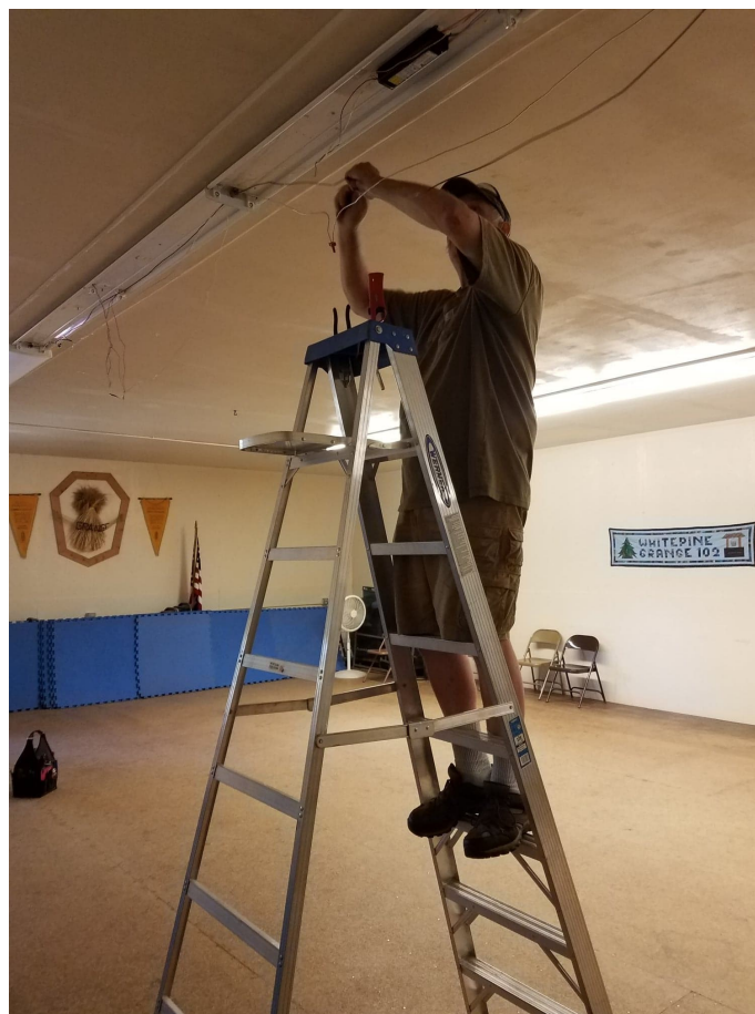
Above: Volunteer Mike Bingham installs the new LED light fixtures in the main hall, replacing the old fluorescent tubes. A rebate from NLI helped pay for the new lights.
