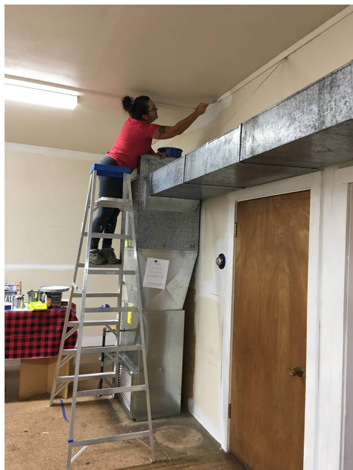
Above: Volunteer painter Nan Blake was not afraid to climb high to the hard-to-reach wall sections around ductwork.
